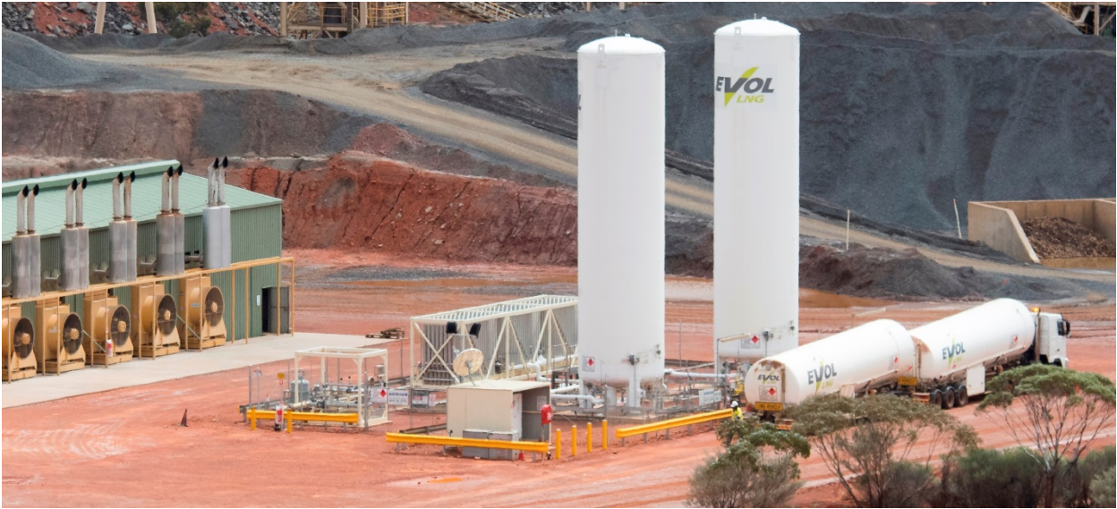
Photo: A typical EVOL LNG storage and vaporisation facility located in the Goldfields region of WA
